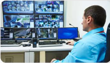
Security Surveillance System
